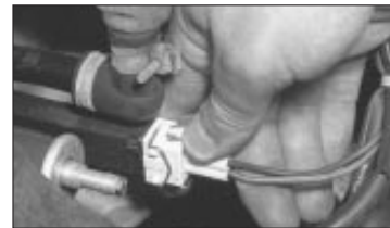
E Wiring plugs may cause problems if dirty or not connected properly.
